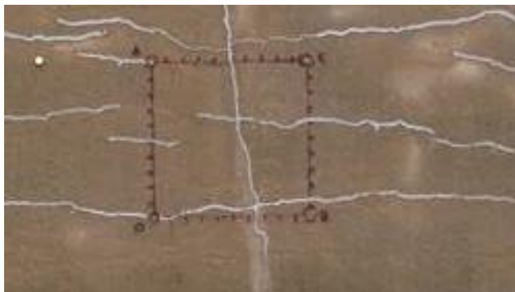
Fig. 3.3-3 —Typical strain measurement grid on barrier section after treatment with silane (by Richard Deschenes Jr.).
