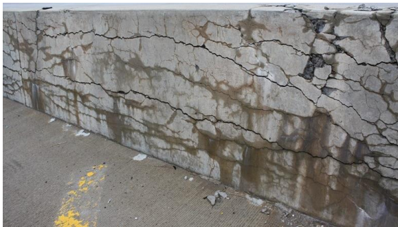
Fig. 3.3-1 —Typical barrier section with severe damage (by Richard Deschenes Jr.).
