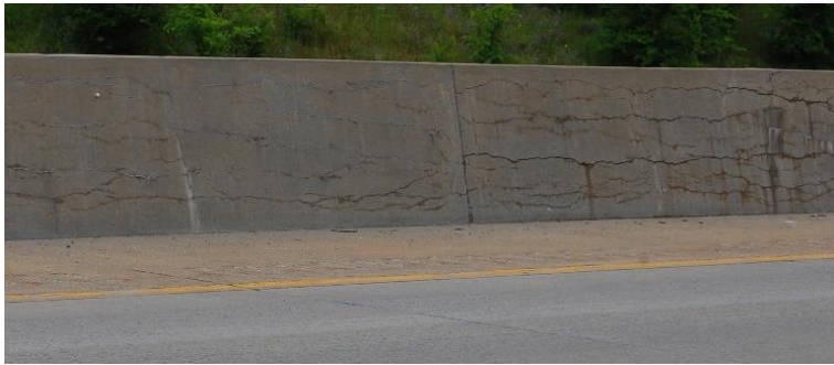
Fig. 3.5-4 —Silane-treated section (left) as compared to untreated section (right) (by Richard Deschenes Jr.).
